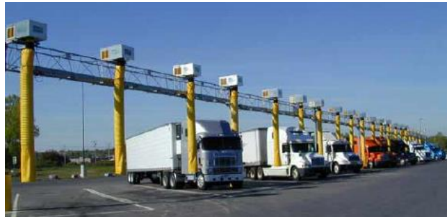
Figure 2 – Service area with a shore power system. [3]
